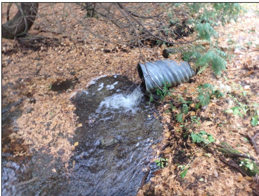
Photo 12: Photo showing the perched CSP and plunge pool at the pond outlet (Photo Date: October 22, 2020)
