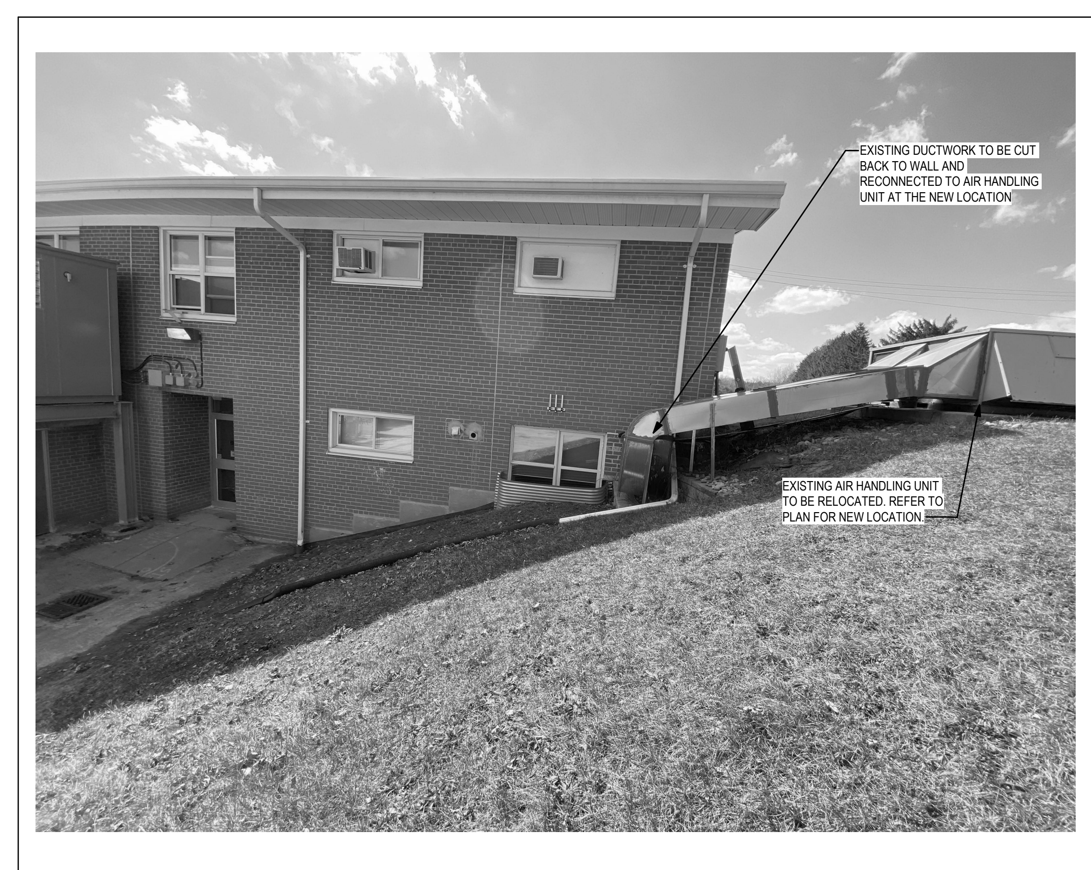
3 PHOTO OF EXISTING AIR HANDLING UNIT M102E SCALE: 1:1
